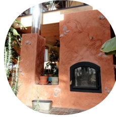
Picture 36: Masonry heater
