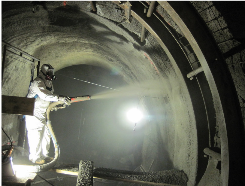
Figure 3.7: Shotcrete applied on steel reinforcement arches in access tunnel (Shotcreting Over Steel Ribs in Preparation for Waterproofing in Access Tunnel 4 (3-23-11), by MTA Construction and Development, 2011, Flickr, ( https://www.flickr.com/photos/59595815@N03/5557948927 ). CC.)
