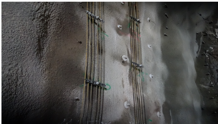
Figure 3.13: Photo of reinforced rebar arches before being covered with shotcrete (photo received from expert at the E4 Stockholm bypass project).
