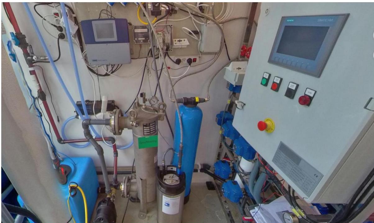
Figure 13 showing an inbuilding greywater treatment system installed in HSB LL.
