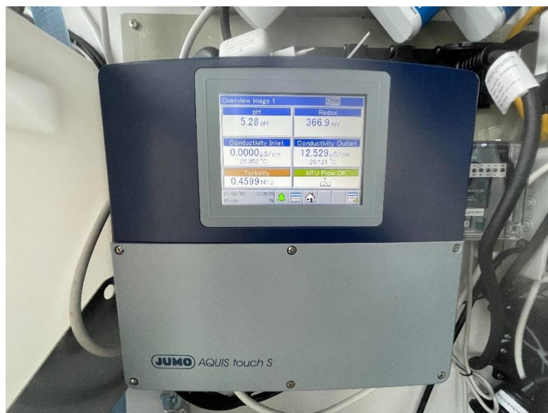
Figure 20 showing physical parameters monitoring sensor installed in HSB LL.
