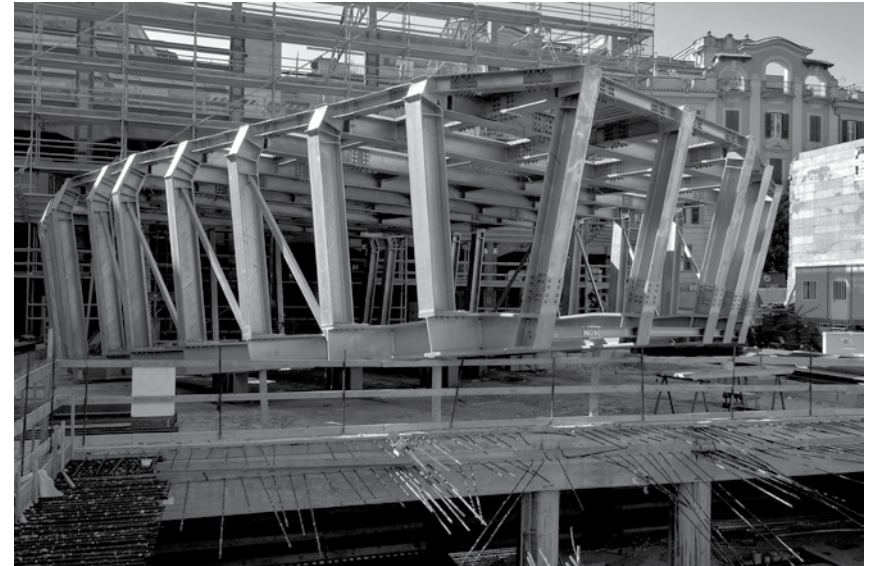
The construction of the red polygon in the middle of the entrance hall. (photo by: Alessandro Di Silvestre)
