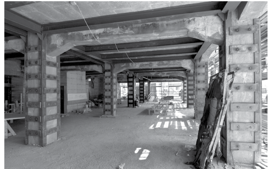
The old building facing Via Nizza was chosen to be renovated and reused. The pillars had to be reinforced and a steel construction was created around them. (photo by: Alessandro Di Silvestre)
