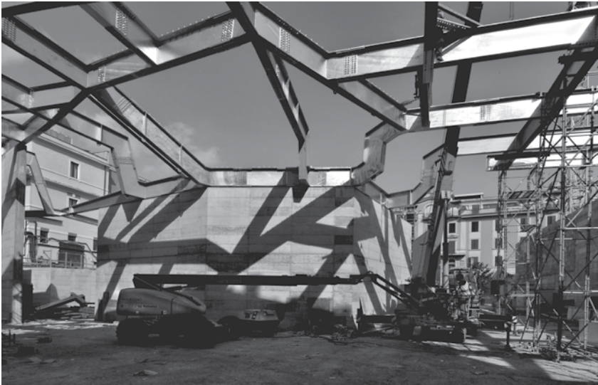
The construction of the roof over the new entrance hall. (photo by: Alessandro Di Silvestre)
