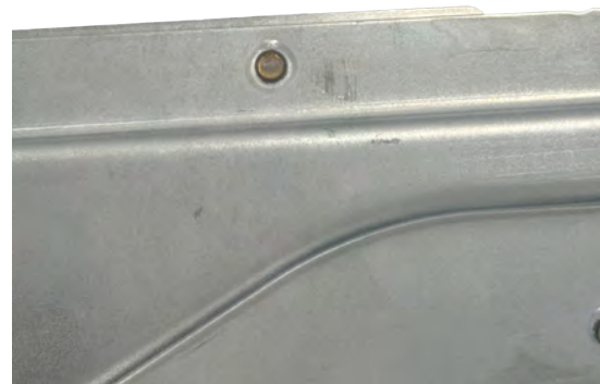
Figure 4.46: Closeup of the physical assembly showcasing a mismatch between the flanges at a joining location.
