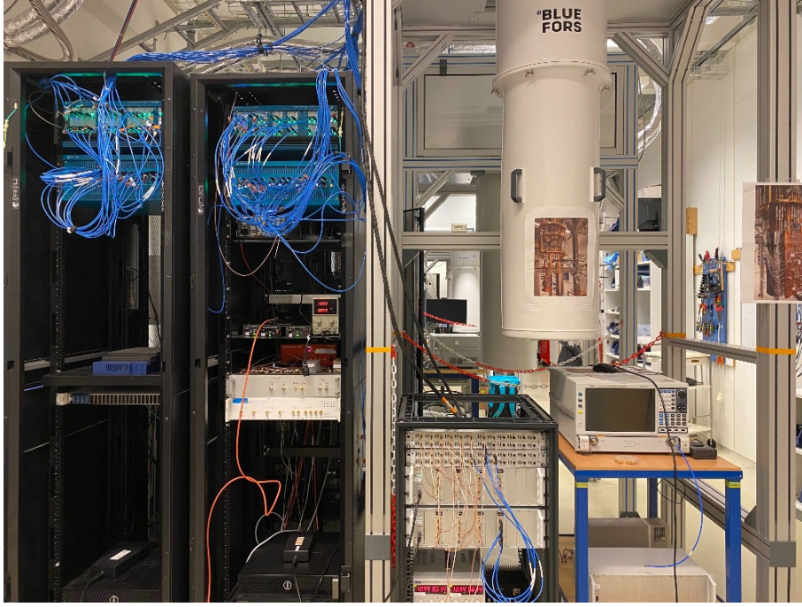
Figure 3.5: The experimental setup. A photo of the cryogenic measurement setup showing the Bluefors dilution refrigerator (right), Qblox clusters (left), other electronics, and cables.
