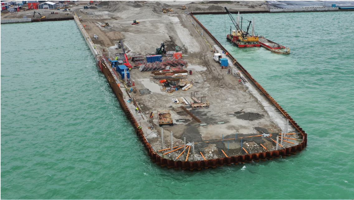
Figure 3.2: Installed sheet piles, the production of the capping beam has started (PEAB, 2021).
