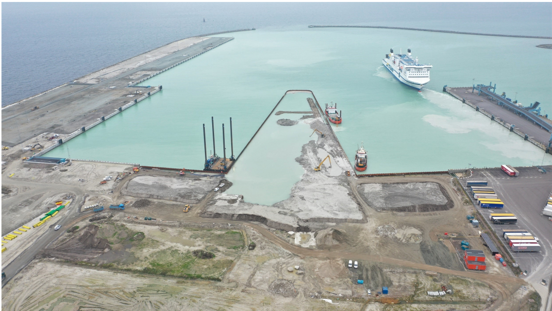
Figure 3.1: Picture taken during construction of the project for the case study (PEAB, 2021).
