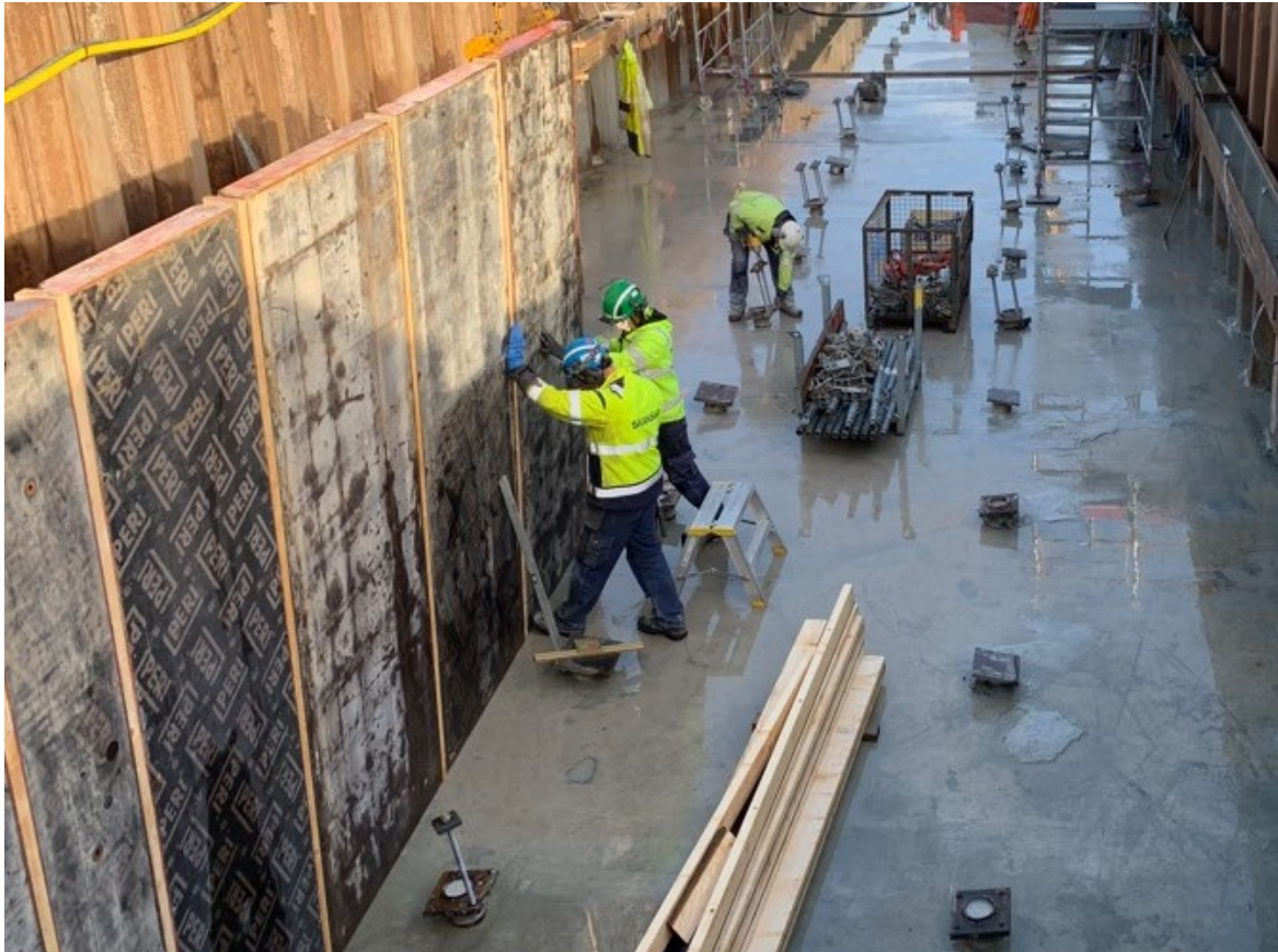
Figure 2.6: Picture from the erection of the new retaining wall structure at Packhuskajen (Sweco AB, 2020).
