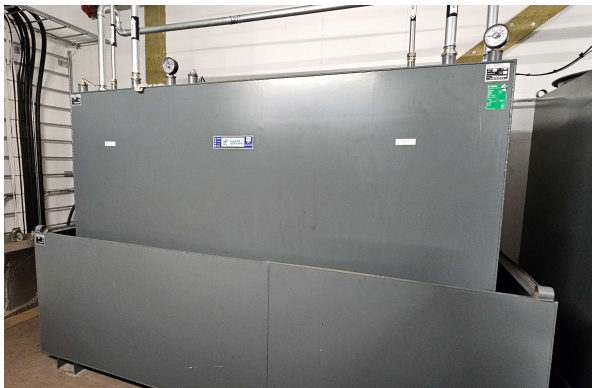
Figure 14: Cistern where the waste oil is collected.
