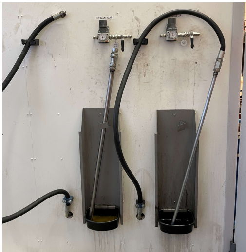
Figure 13: Arrangement on the wall where the engine oil is sucked up to the cistern.
