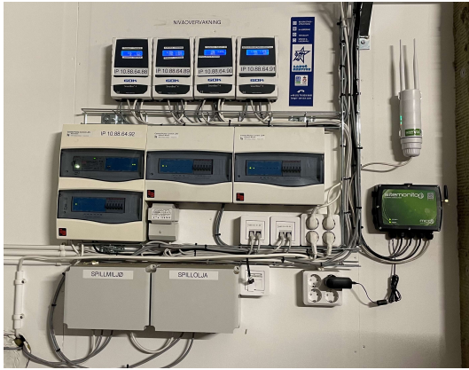
Figure 15: Panel where the level sensors are connected to.
