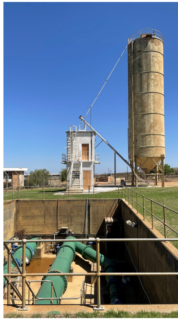
Figure 3.7: Lime storage and dosing at Withoogte DWTP.
