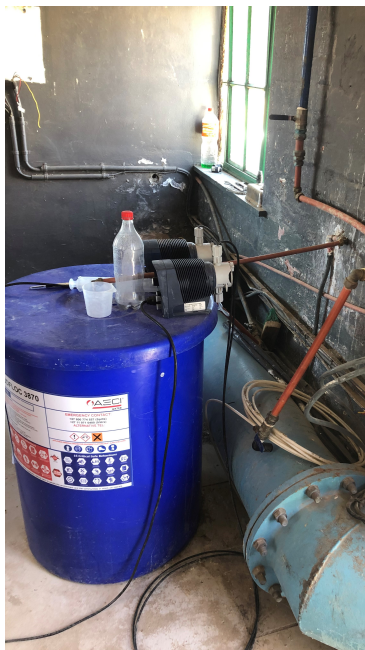
Figure 3.2: Addition of coagulant at Piketberg DWTP.
