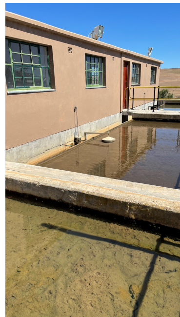
Figure 3.4: Rapid gravity sand filter at Piketberg DWTP.
