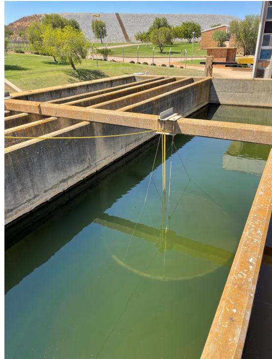
Figure 3.10: Vertical sedimentation at Withoogte DWTP.
