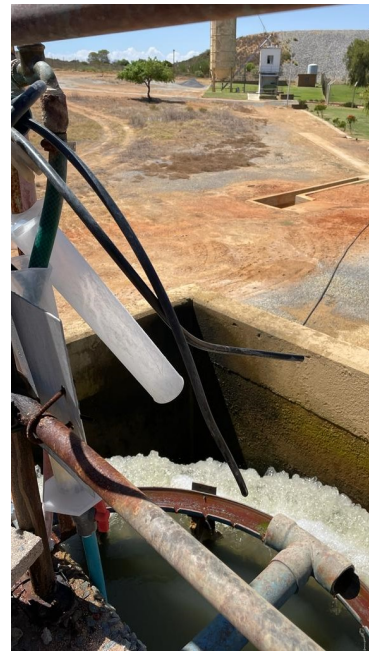
Figure 3.8: Dosing of the coagulant at Withoogte DWTP.
