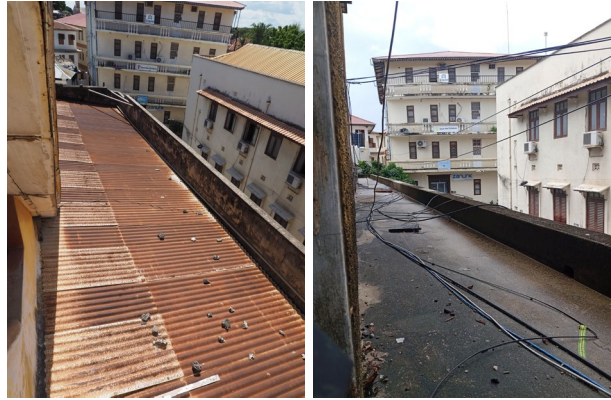
Fig65. The existing conjugated metal surface
