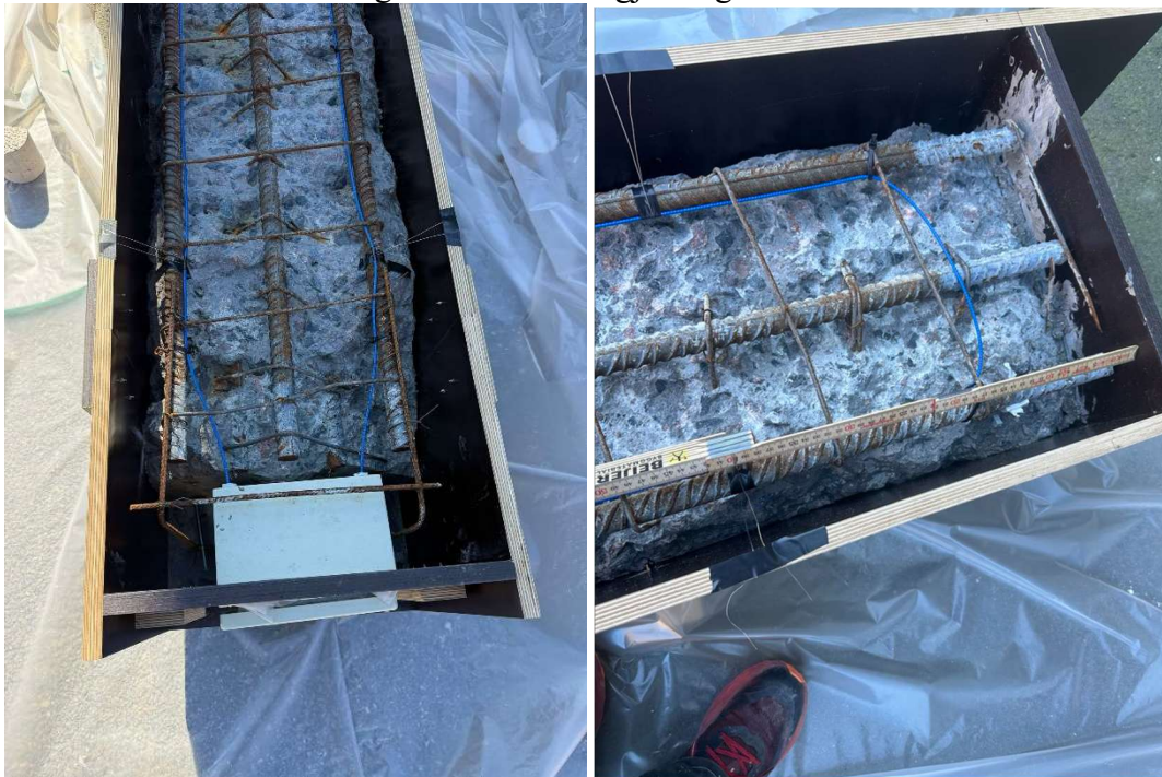
Figur 7.7: Fiberoptikinstallation (Egna bilder, 2025)
