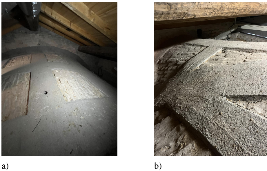
Figure 3.11: Pictures of current state of the TRM application on St. Bassiano, a) Barrel vault and b) Ribbed vault.
