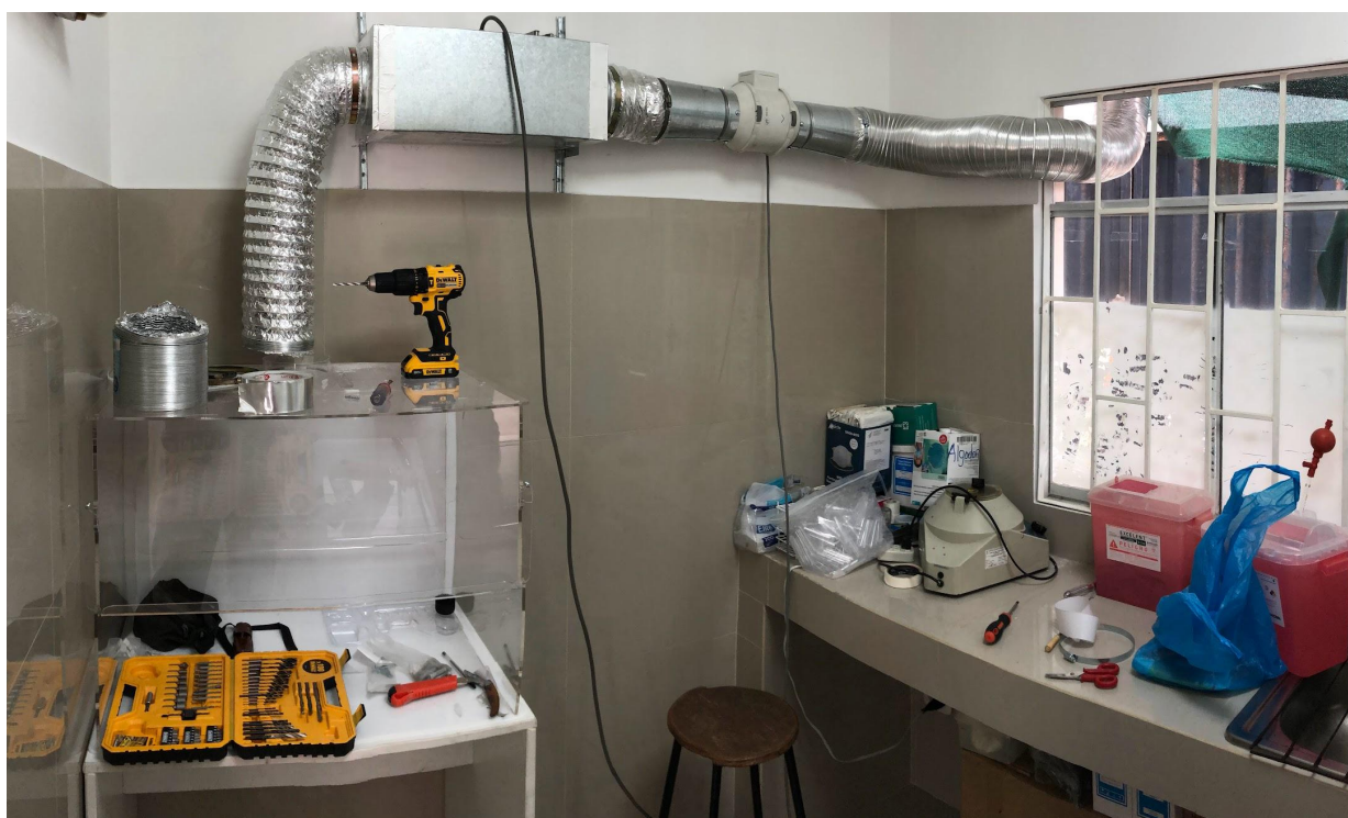
Figure 3.42 Old dysfunctional cabinet (top), in the progress of setting up the first iteration of the FVWS for real-world use (bottom)
