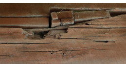
Rafter (need to be repaired) 220 x 120 mm x 2
