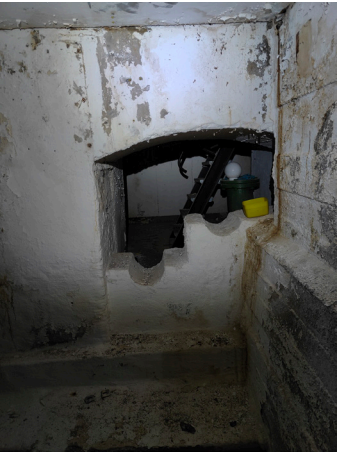
Figure 51. 26. Hole in wall and damaged surface layer
