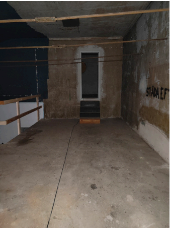
Figure 37. 14. Loose tie rods and height differences
