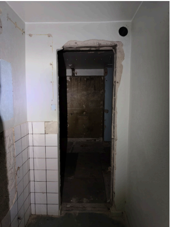
Figure 46. 22. Damaged tiles and door opening
