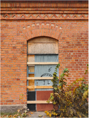
Figure 33. 11. Wooden door with broken glass partitions
