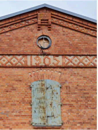
Figure 34. 12. Damaged window frame and rusty shutters
