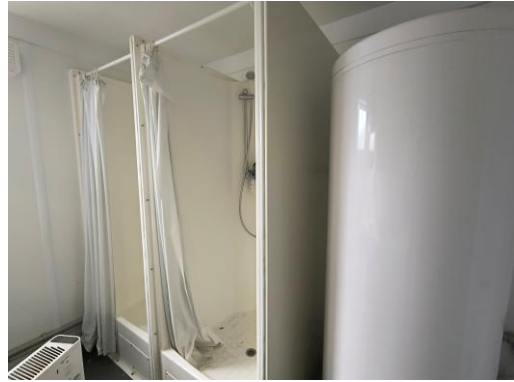
Figure 4: Showers in the sanitary container on site 1. (Picture taken by the author)
