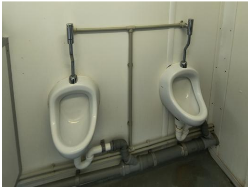
Figure 5: Urinals in the sanitary container on site 1. (Picture taken by the author)
