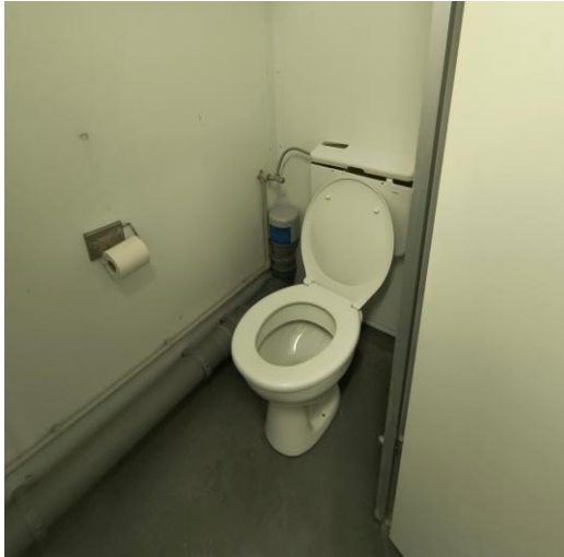
Figure 3: One toilet in the sanitary container on site 1. (Picture taken by the author)
