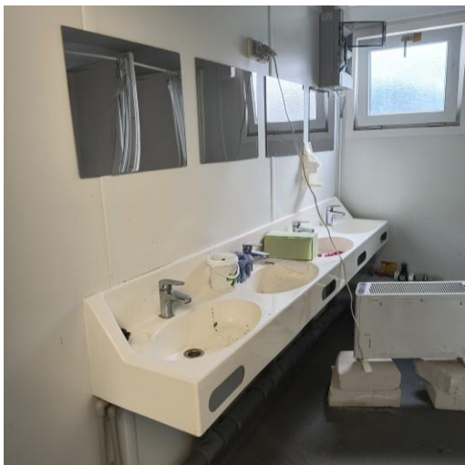
Figure 7: Sinks in the sanitary container on site 1. (Picture taken by the author)
