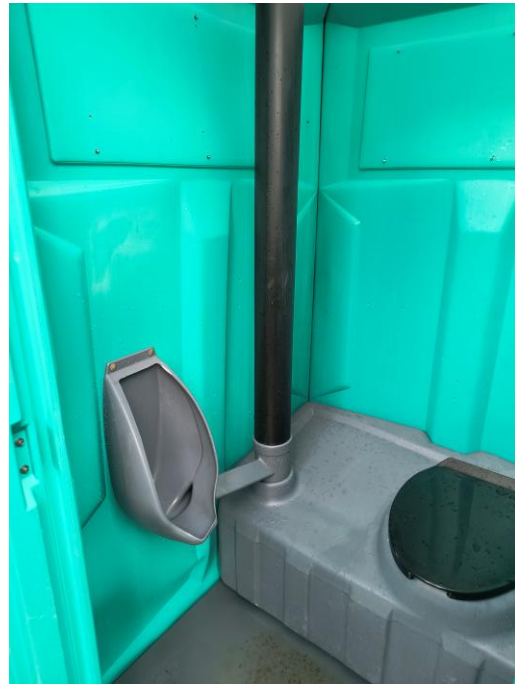
Figure 14: Portable toilet from the inside on site 3. (Picture taken by the author)
