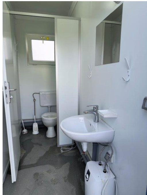
Figure 12: Women's toilet in the sanitary container on site 2. (Picture taken by the author)
