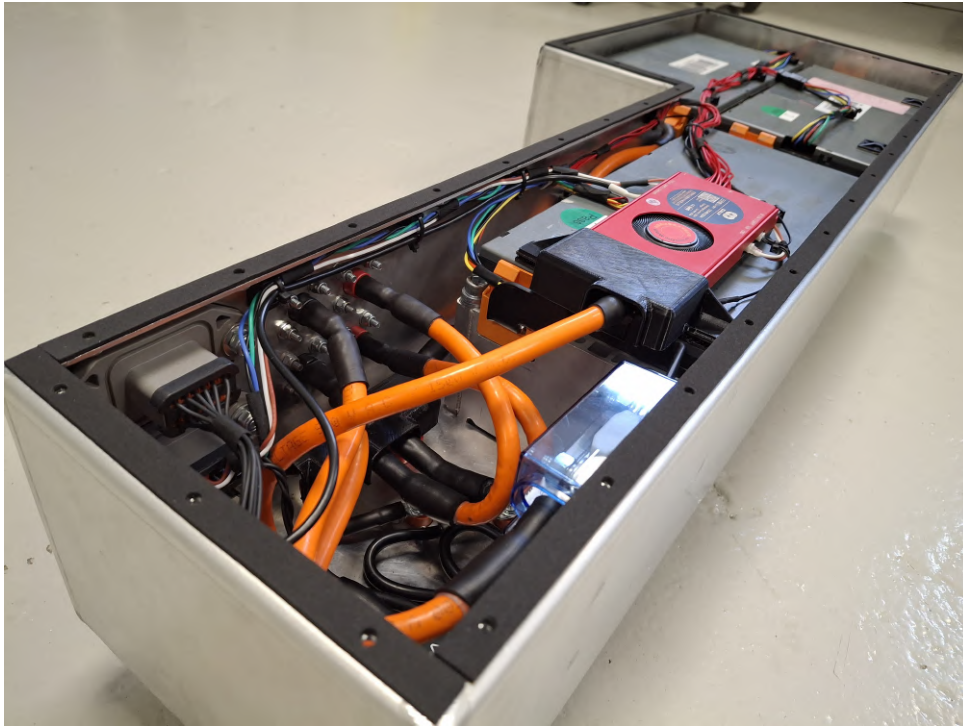
Figure 6.5: Finalized internal battery cable routing
