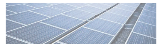
Figure (52) Solar panels
