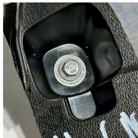
(b) Close-up of physical joint.
