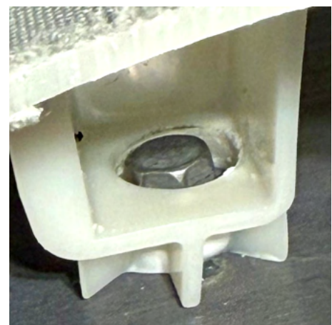
(b) Close-up of physical joint.
