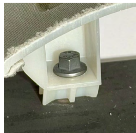
(b) Close-up of physical joint.
