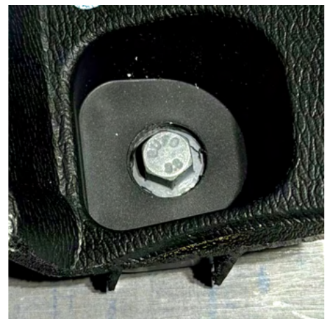
(b) Close-up of physical joint.
