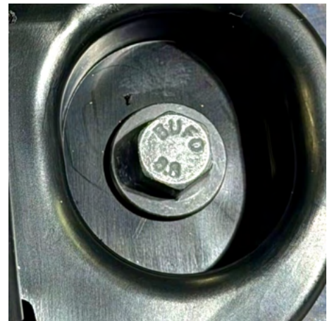
(b) Close-up of physical joint.
