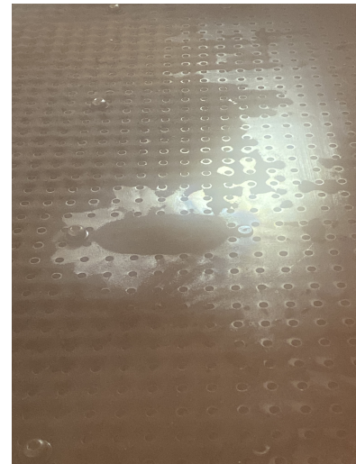
(b) Abrasion caused by cyclone.
