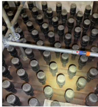
Figure A.1: Perforated nozzles that provide primary air in Amagerværket, provided by HOFOR.
