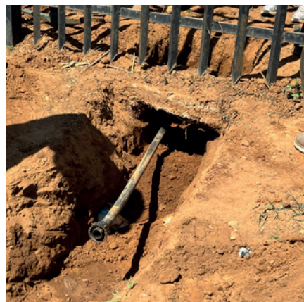
The broken and exposed pipe
