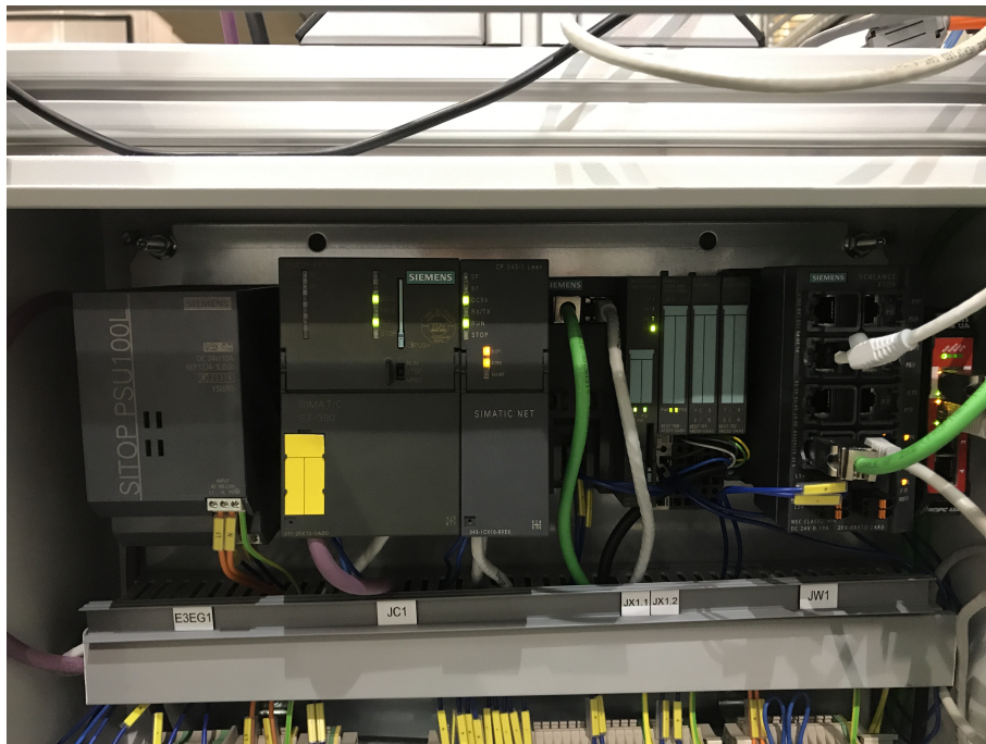
Figure 5.1: Zoomed picture of the components installed in the PLC cabinet
