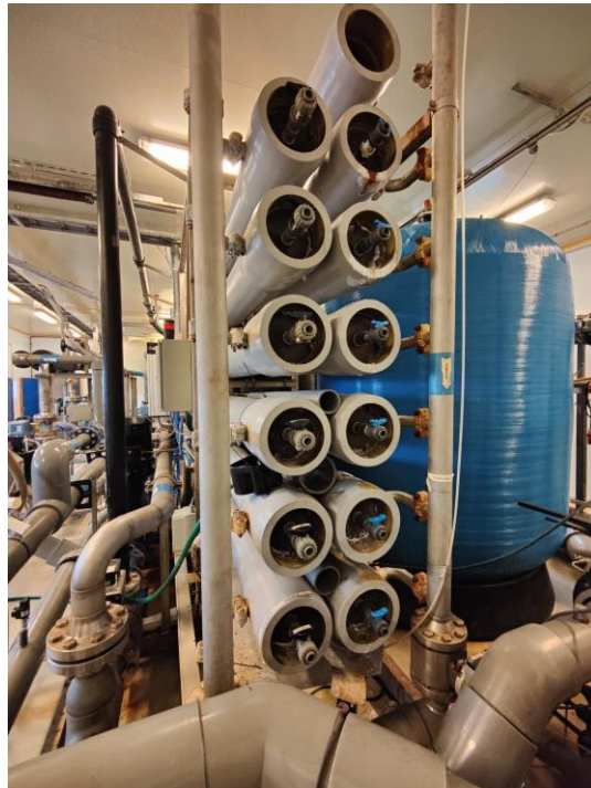
Figure 3-1: RO membrane units in Galtneset
