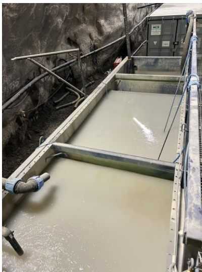
Figure 16. The pH regulation container (Photo by the authors).
