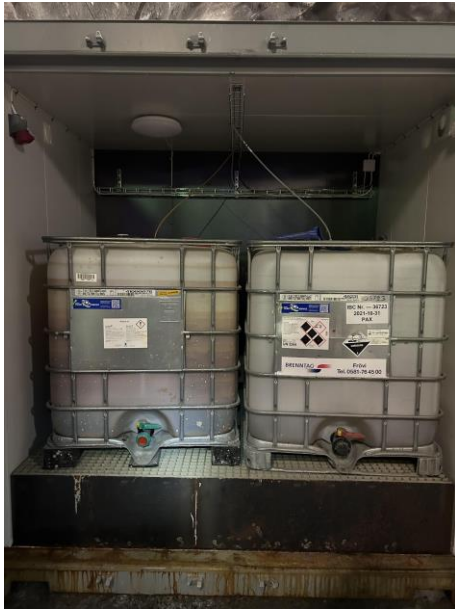
Figure 19. PAX and RedOx flocculants dosed from IBC containers (Photo by the authors).
