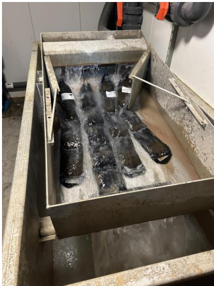
Figure 17. Chitosan socks inside the Hydrobox (Photo by the authors).
