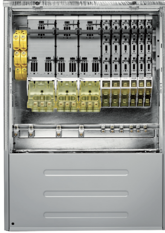
Figure 3.2: Internal structure of the AC distribution cabinet.
