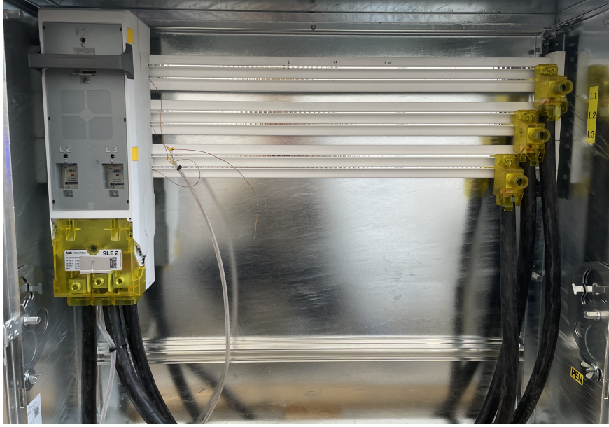
Figure 4.7: AC Cabinet Components
