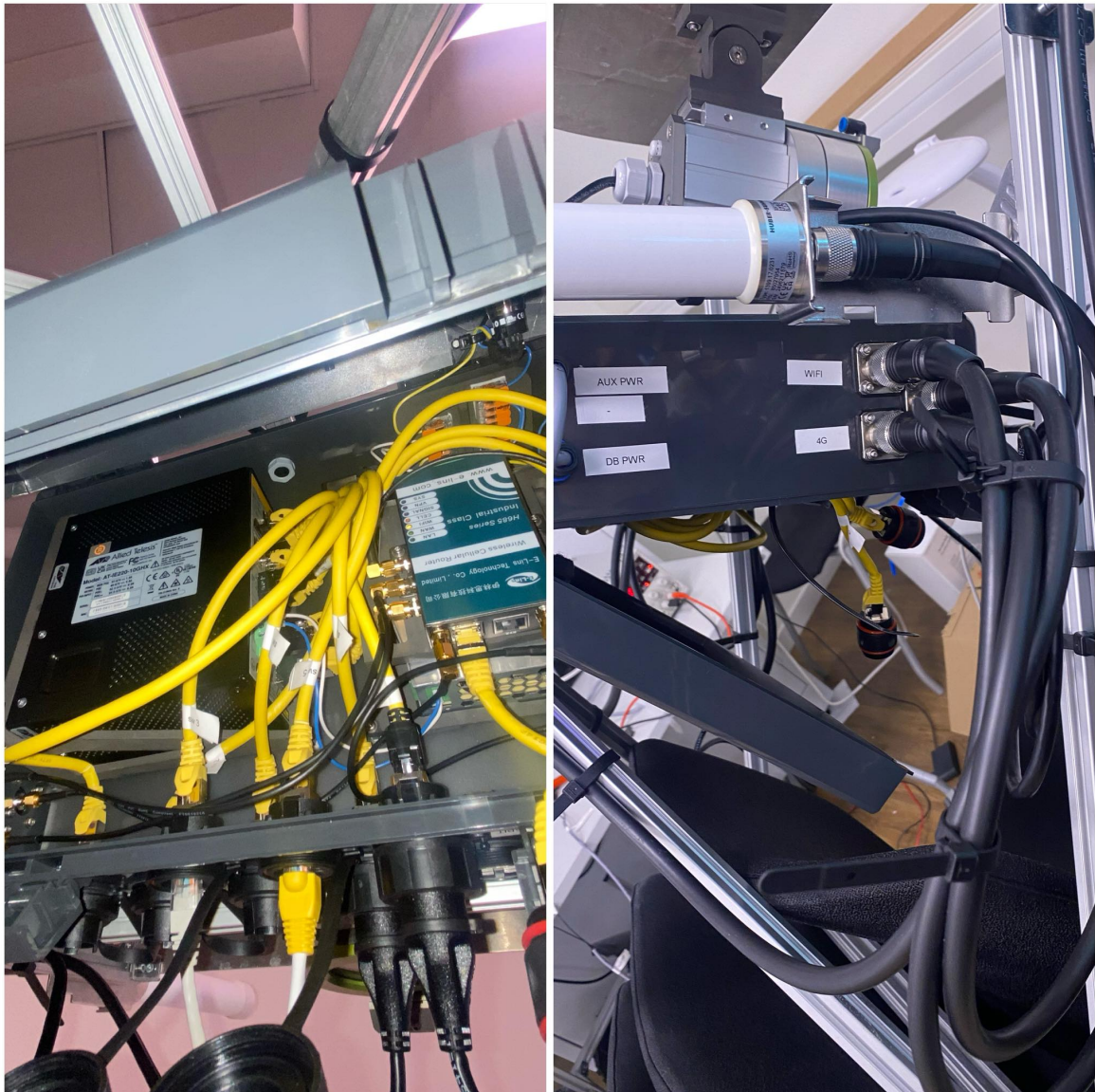
Figure B.4: The components within the case in an upside down position
