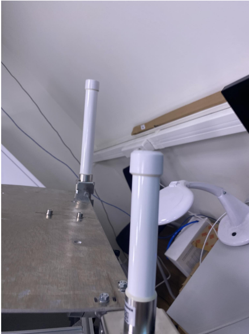
Figure B.5: 4G/LTE and Wi-Fi antennas installed in the small white tubes
