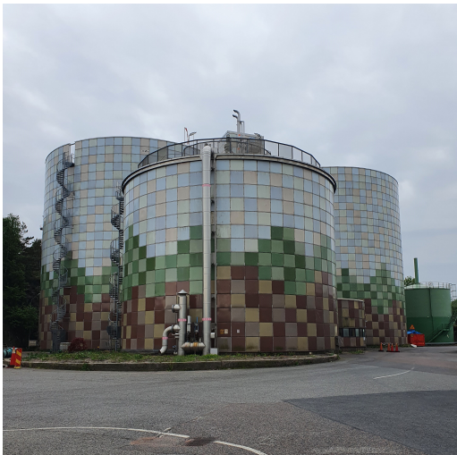
(a) Digestion chambers
