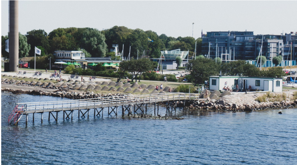
Doppingarna's temporary structure on the site of the former bathhouse after the storm.
