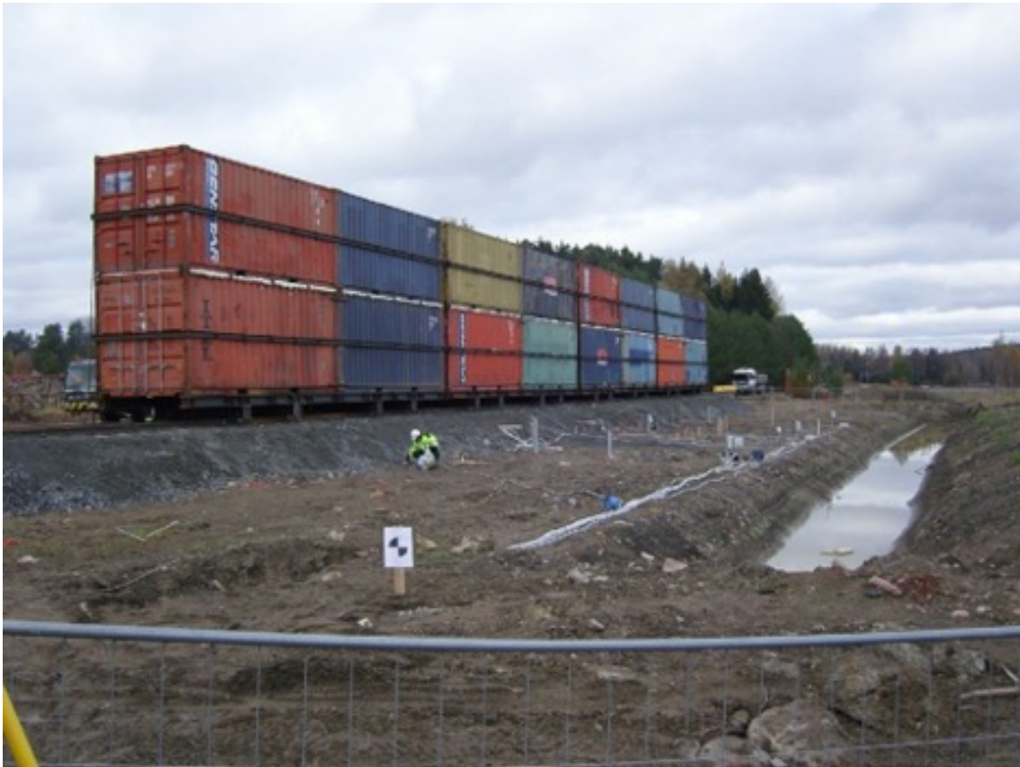
Figure 3.2: Photo taken at the Perniö test site, before failure (Mansikkamäki, 2015).
