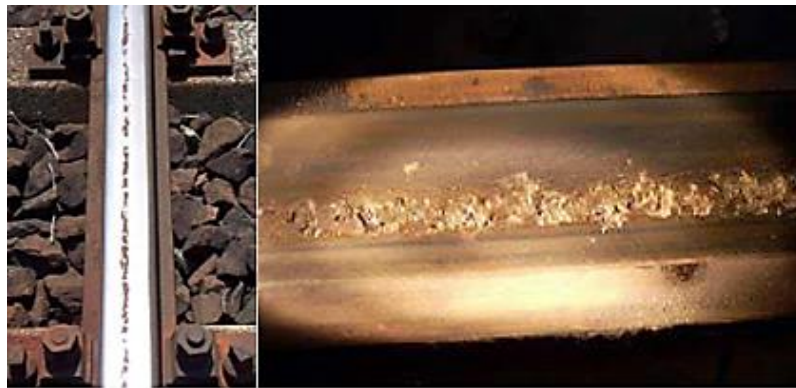
Figure 12: Spalling on the rail head surface (from [29])
