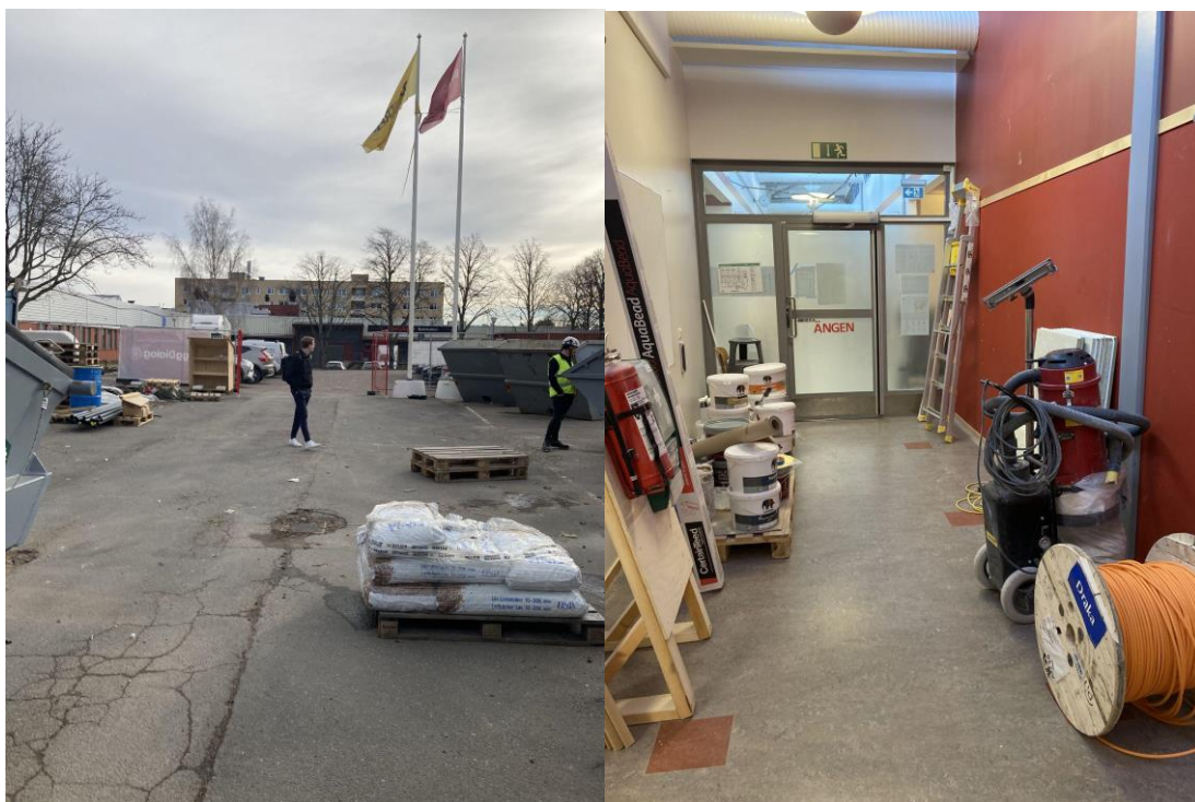
Figure 4.3 Area for deliveries (left) and material storage in corridors (right) (Authors' own figure).
