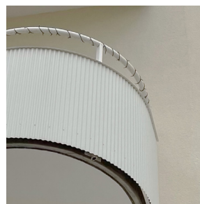
Fig. 4. Balcony railing, Viken. Fig. 5. Balcony railing, Malmö. Fig. 6. Balcony slab panelled in wood, Gothenburg. Fig. 7. Balcony railing and slab, Gothenburg.
