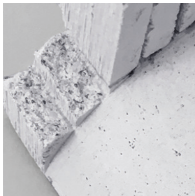
Unintended broken pieces.
