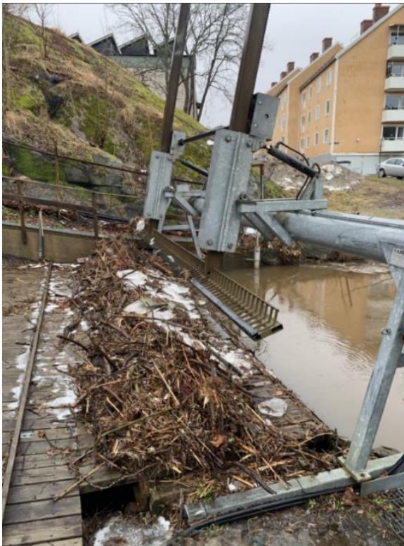
Figure 6. Branches and leaves at the intake gate with automatic cleaner.
