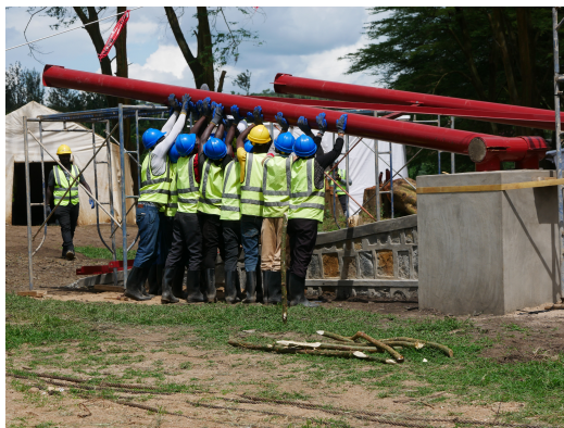
(a) A picture showing a construction site in Rwanda. (Bridges to Prosperity, 2023a). Reprinted with permission.
