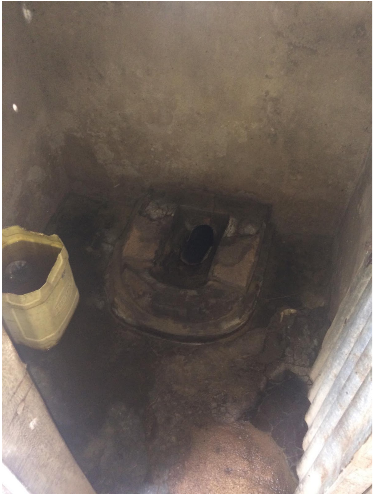
Figure vi. Picture from inside one of the female toilets showing uneven floor, lack of light and water for flushing and cleaning.
