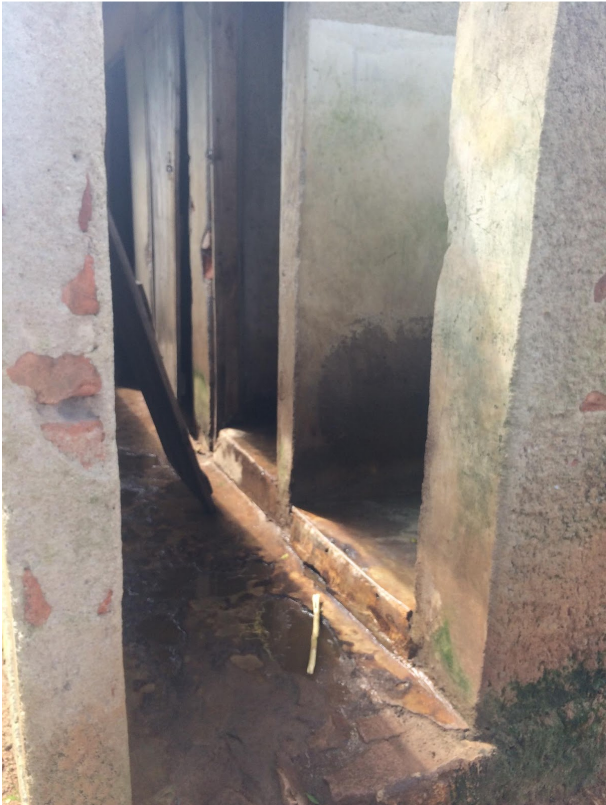
Figure v. The male toilets, missing doors and uneven floors.
