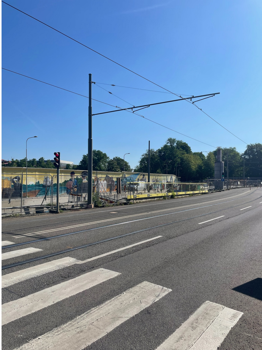
Figure C.2: Photograph (A) of Parkgatan showing a part of the ongoing construction project.
