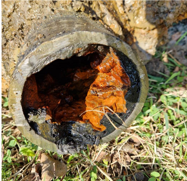
Figure 12: Biofilm buildup in the cut section of the pipe during repair work
