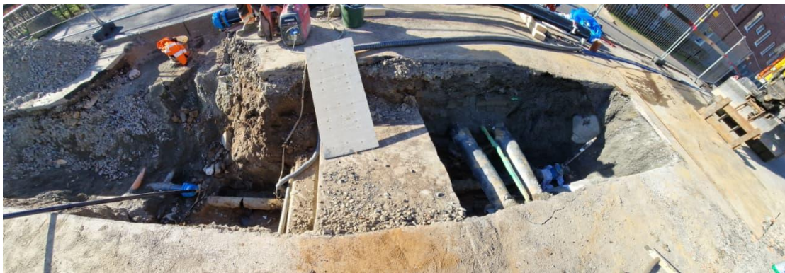
Figure 19: Connecting currently in usage pipe section with already existing unused pipe section
