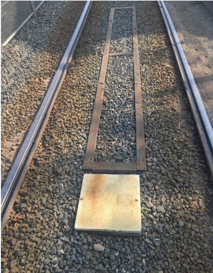
Figure 2. Installation of detector loop for trams on wooden frame including junction box (Göteborgs Stad, 2023) (Photo: Andreas Larsson).
