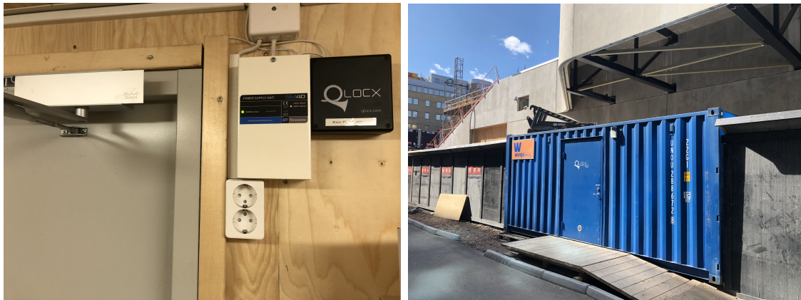
Figure 4.4: Qlocx digital lock inside the container(left) & Qlocx delivery container placed in site perimeter(right) (own images).
