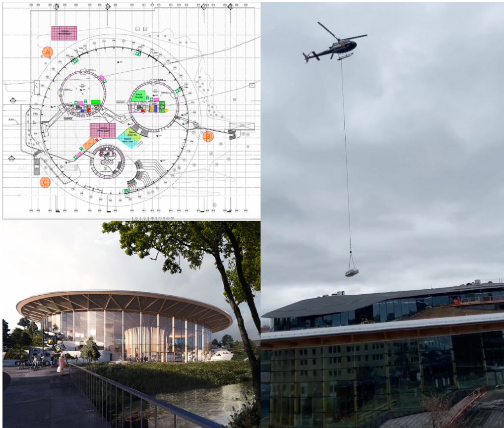
Figure 4.7: Project A: Internal WAP of the third floor (top left), digital rendering of the construction (bottom left) & material handling from the unloading zone to the roof by helicopter (right). Images provided by BRA.
