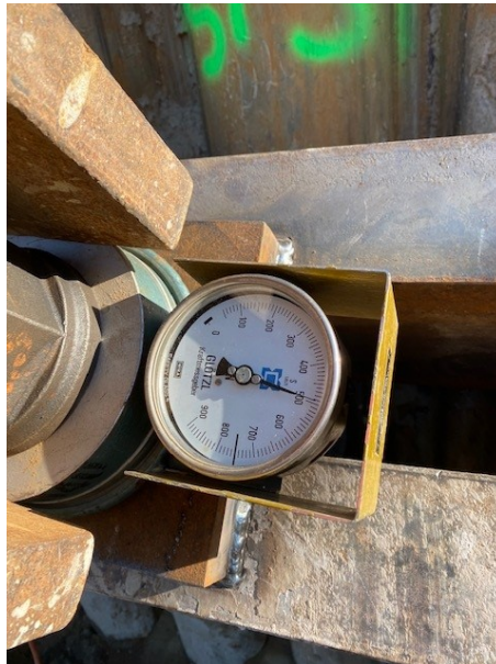
Figure 4.7: An installed ALC, from studied site.
