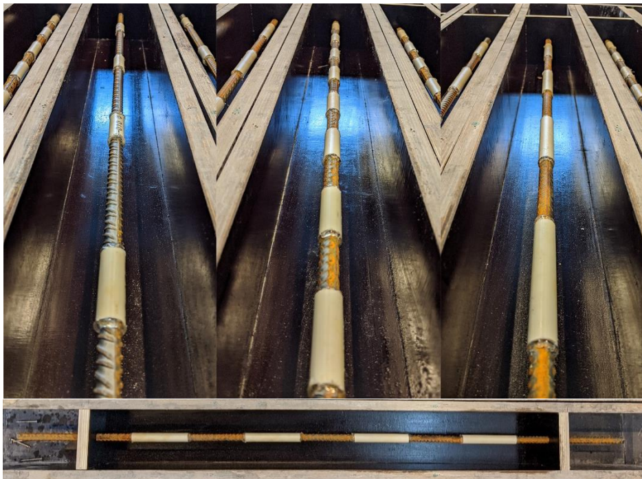
Figure A.4 Installation of three different PVC configurations- 4x50 mm (left), 8x50 mm (center), 4x100 mm (right). The bottom image displays a prism with 4x100 mm ready for casting from a top-down view. Note the spacing between PVC segments and from the wooden ends.
