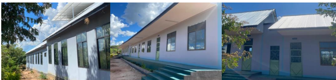
Figure 5.6: Visualisation of the gap and height differences between the two roofs on the school building. a) The facade on the west side. b) The facade on the east side. c) The gap shown from another perspective on the east side. The southern roof is visibly higher elevated than the northern roof.
