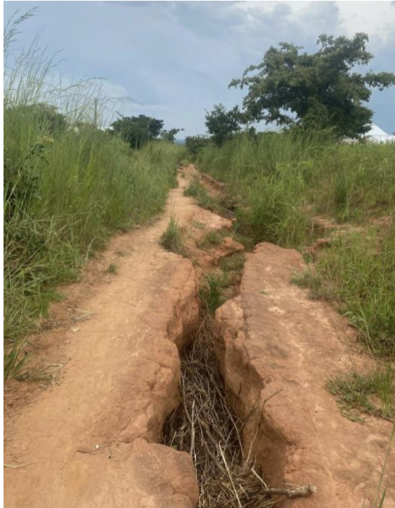
Figure 2.3: Road damaged though soil erosion caused by heavy rain.
