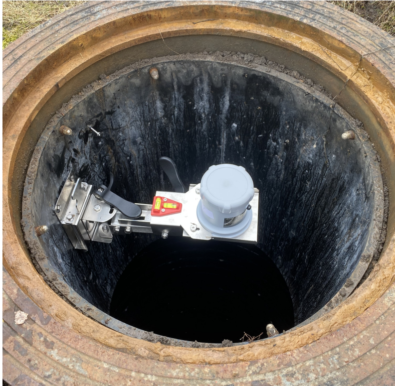
Figure 3.2: Sensor installed by VA SYD.
