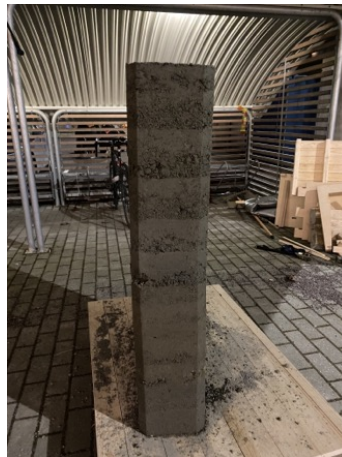
(b) Wall from the side. The upper part is slightly tilted due to formwork not being completely vertical.
