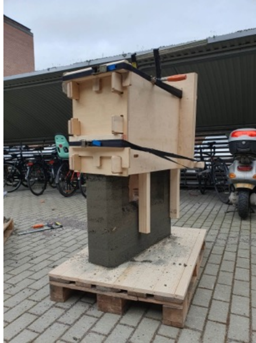
Figure 2.2: Picture showing formwork developed by EarthLAB Studio in use. The form can be moved upwards and sideways along a wall.
