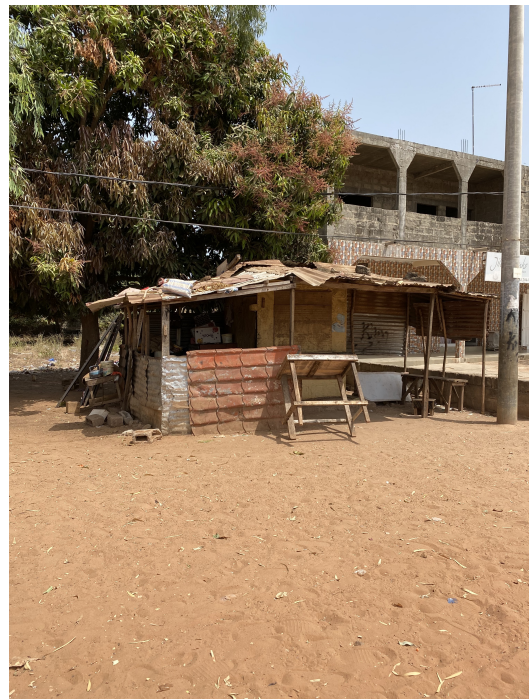
(b) Corrugated steel roof repaired with tart and kept in place with stones.
