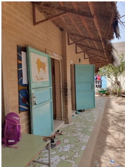
(a) Roof overhang providing shade while the doors to the classrooms are open.
