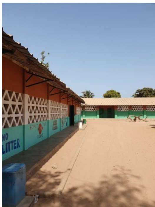
(a) The class room walls are perforated to provide daylight and natural ventilation.
