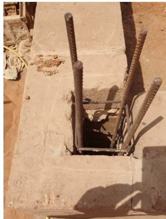
(b) Re-bars prepared for casting concrete pillar with CEB as lost formwork.
