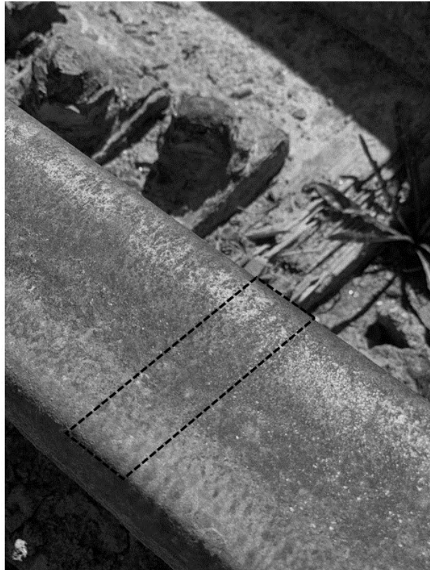
Figure 2.8: Weld between turnout and rail from a freight railway located outside Gothenburg
