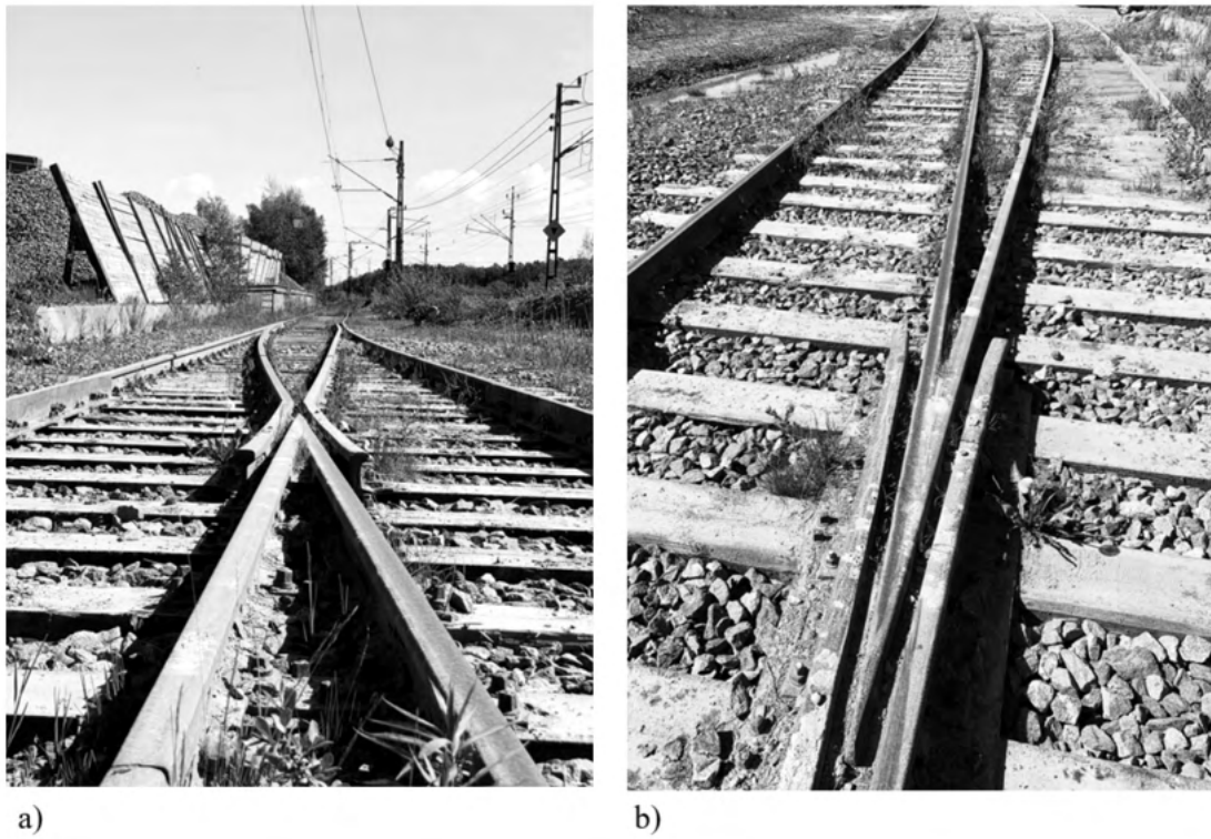
Figure 2.2: Field example of a) a turnout and b) a crossing nose from a freight railway located outside Gothenburg
