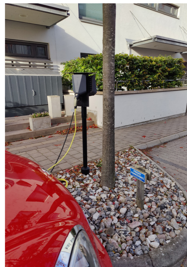
Picture 7. Charging station for electric vehicles.
