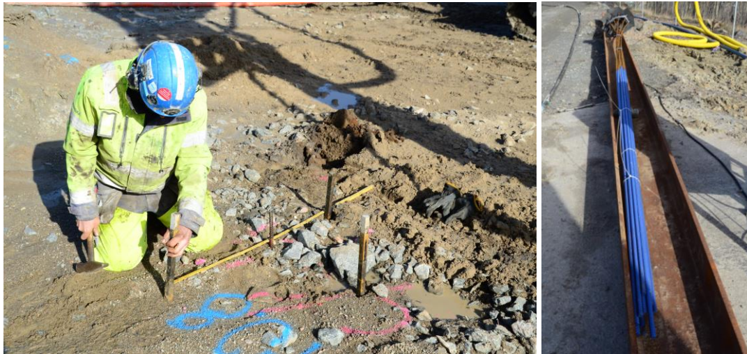
Figure 34 Photographs taken during the painted bars test; measuring and installation (left) and uninstalled bars (right).
