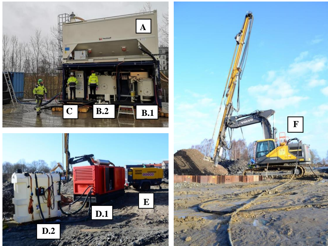
Figure 31 Photographs of the equipment set-up in zone 2 including the three working stations; the mixing plant (top left), the water pump for the drill tip and air compressor (bottom left), and the jet rig (right).
