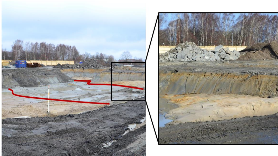
Figure 29 Photograph of early excavation works in zone 2; the layer of clay marked between the red lines and a close-up of the clear distinction of different soil layers at the site. This area is located in between the two test locations.
