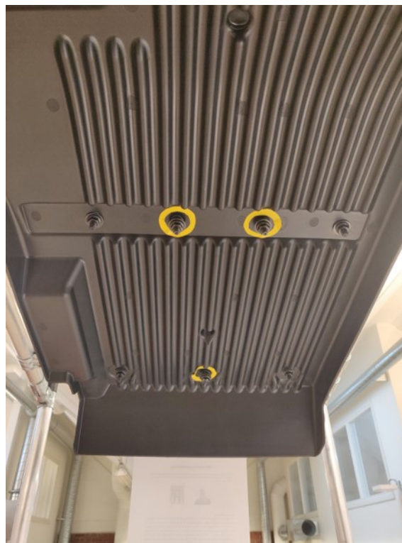
Figure 3.2: Yellow marked bolts
